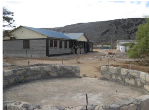
New maternity ward on the left with old dispensary on the right in the distance, taken from the foundation of one of the Manyattas (maternity waiting home)
